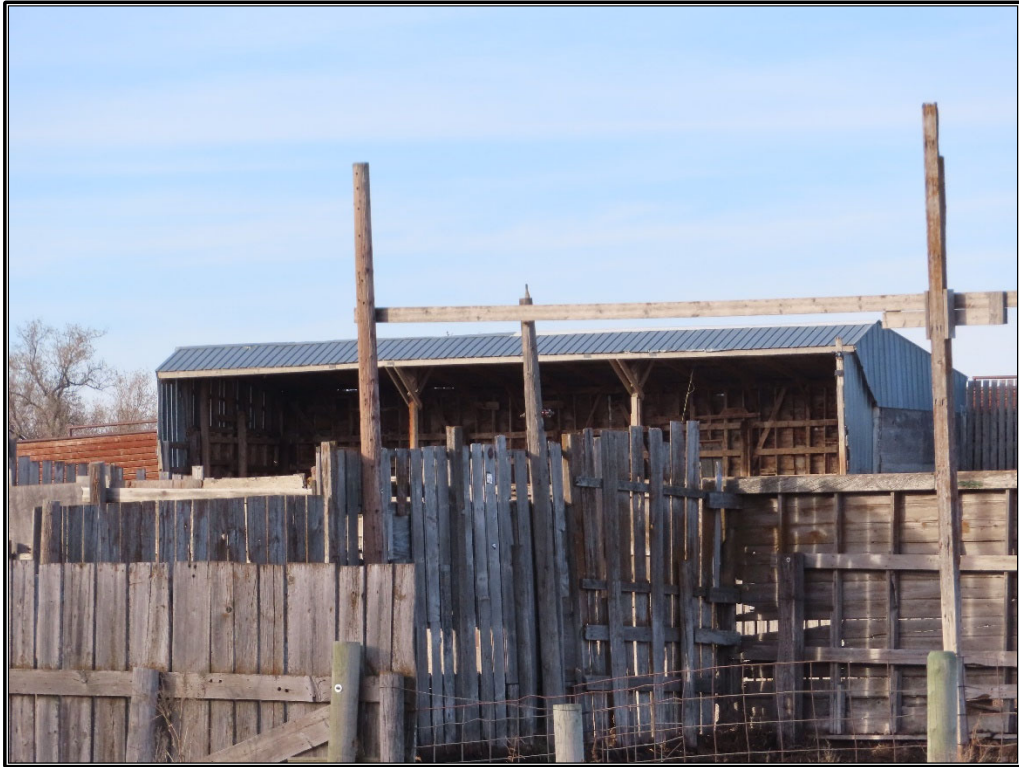
Figure B-57. Site 8: Animal shelter No. 2, south and east elevations, facing northwest.
