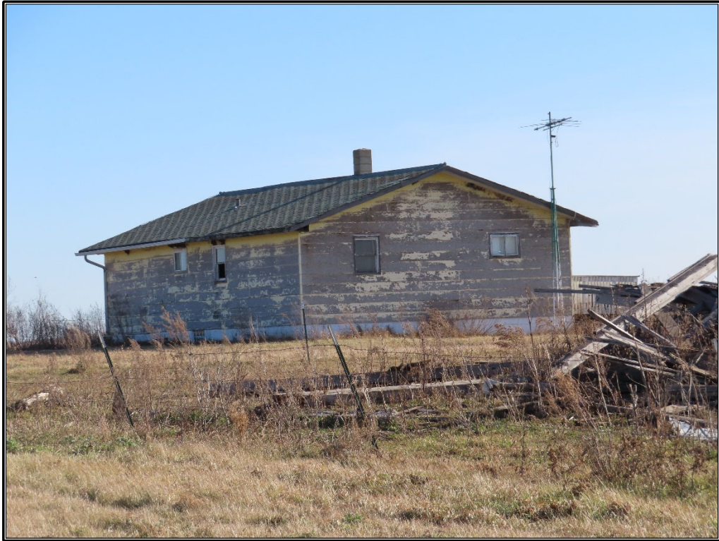
Figure B-15. Site 2: North (rear) and west elevations of residence, facing southeast.
